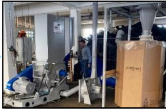
Grinding at sorting location
